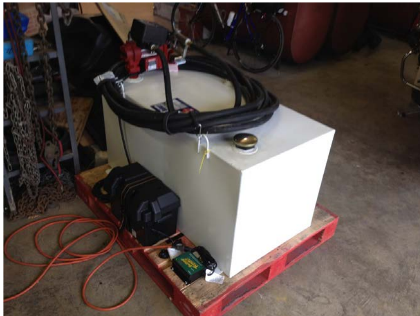
Mobile Fueling System for City Generators
