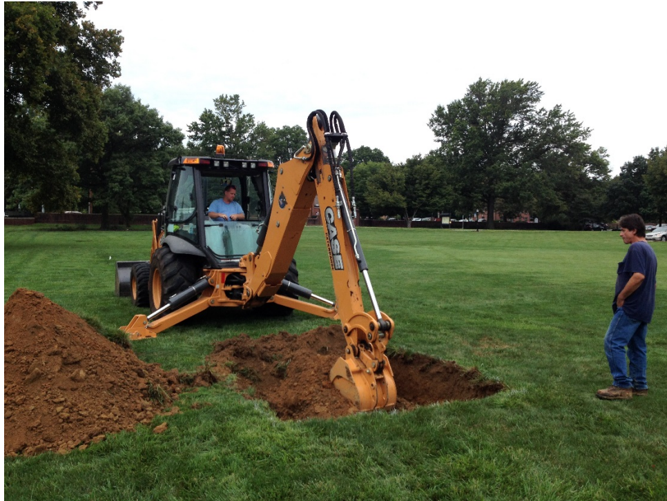
Figure 1: Excavation of storm pipe defects in Laurel Field
